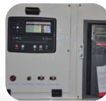
Control Panel & MCB
